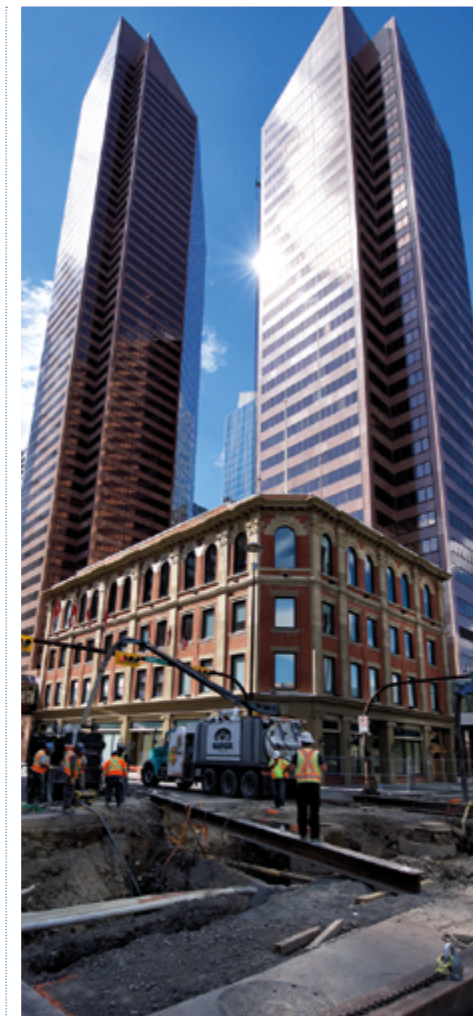
Volker Stevin Canada has begun construction on Calgary's newest office building: TELUS Sky.
