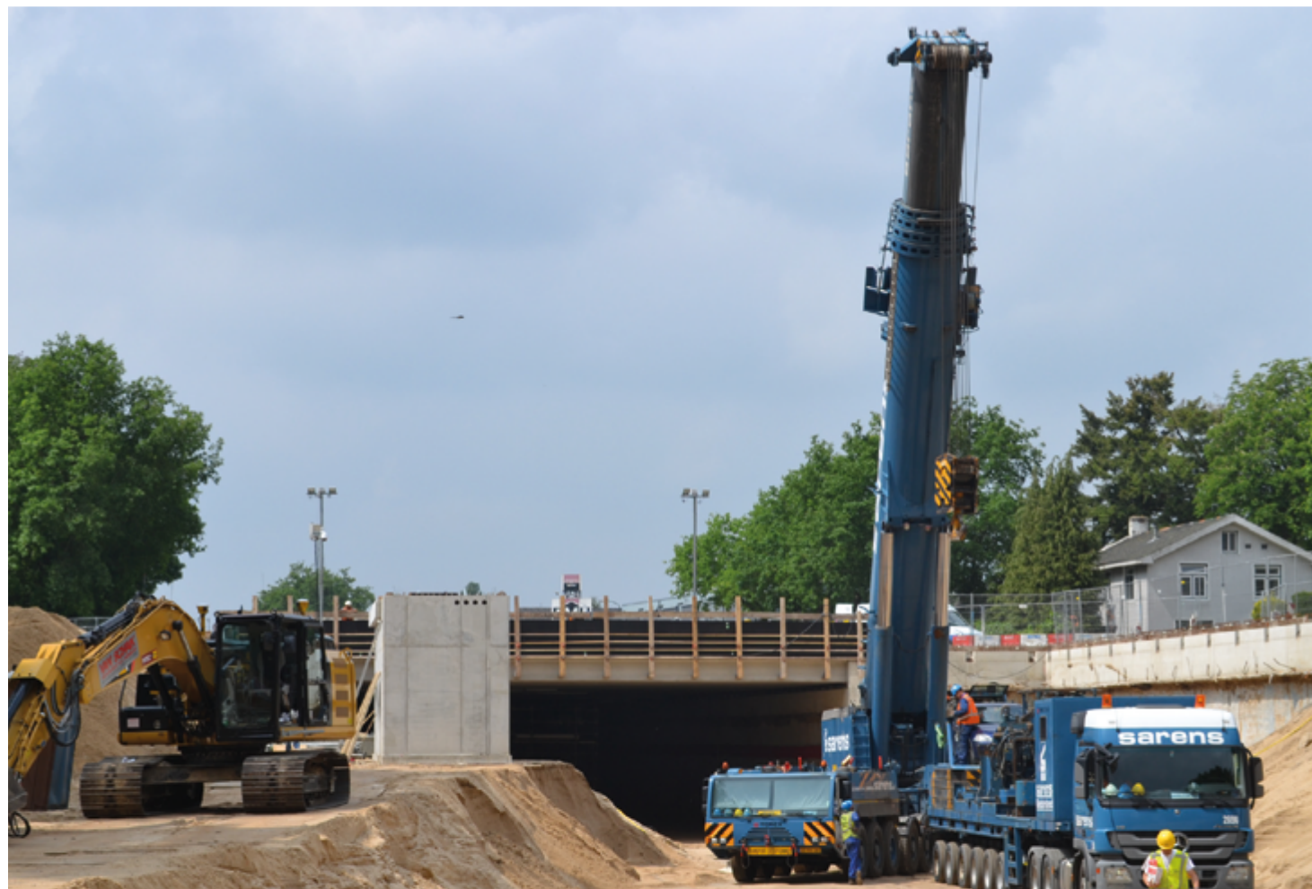
The Combinatie Van Hattum en Blankevoort bv-kws Infra bv consortium has been commissioned by the Dutch province of Utrecht to lower the grade of the N237 provincial road at Soesterberg, where it bisects the town, dividing Soesterberg-Noord from the town centre. Given that the N237 acts as a barrier that hampers not only crossing traffic but also the development of the town as a whole, lowering the roadbed is a crucial subproject within the Soesterberg Masterplan.
