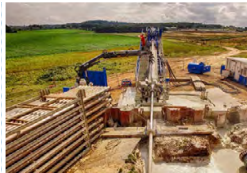
HDD for export cables
