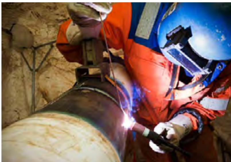
Visser & Smit Hanab maintains the Rotterdam-Beek pipeline (PRB).
