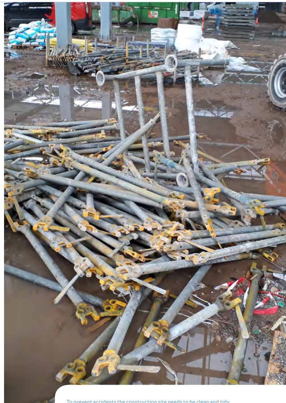
To prevent accidents the construction site needs to be clean and tidy.
