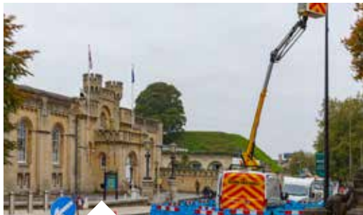
Oxfordshire LED lighting upgrade
