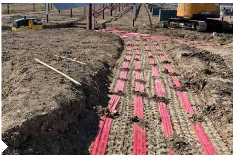
Travers Solar Project
